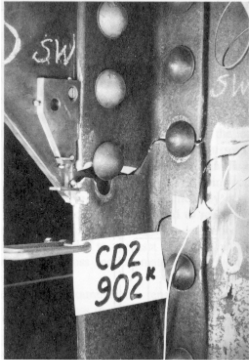
Fig. 6.3. Angle failure in built-up section. (Courtesy of University of Illinois.)
