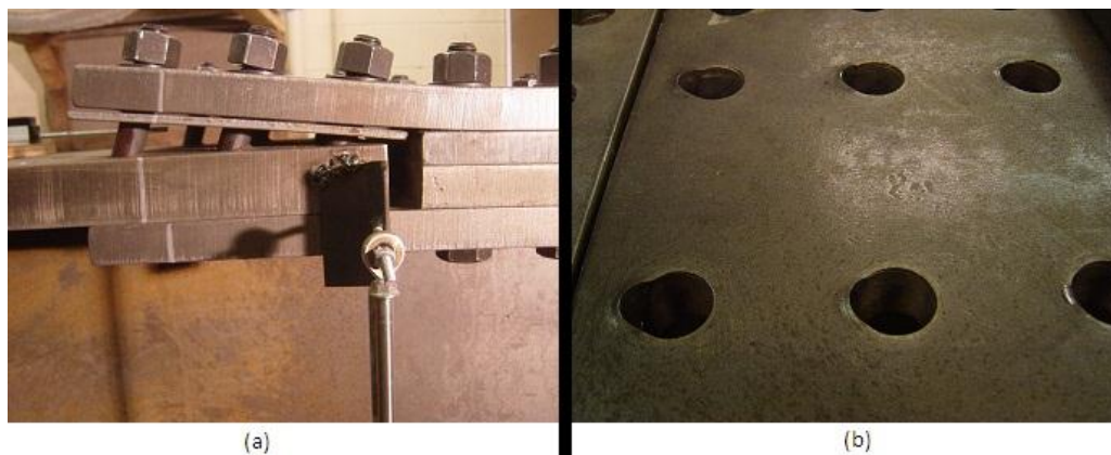
Figure 33: Regions of plastic deformation after girder tests in (a) the top splice plate/bolts and (b) the bolts holes.
